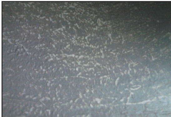
Corroded tank internal surface
